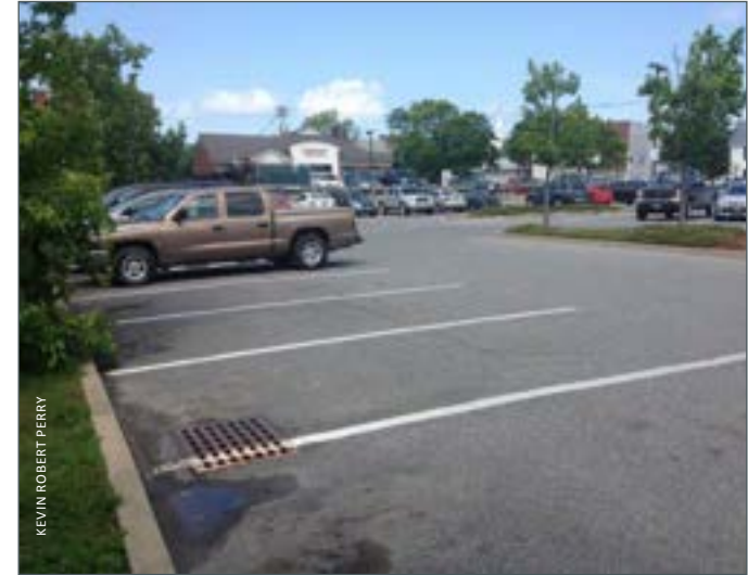
▲ Overly long parking stalls can be shortened to allow for landscaped space at the front of vehicles to capture runoff.
